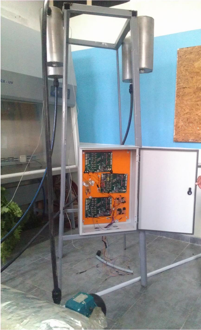
Figure 16.14b: Installed Electrical Control Cabinet
