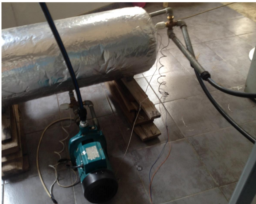
Figure 3.3: The Test 3 concerning open/close 2 valves and turn on/off pump.
