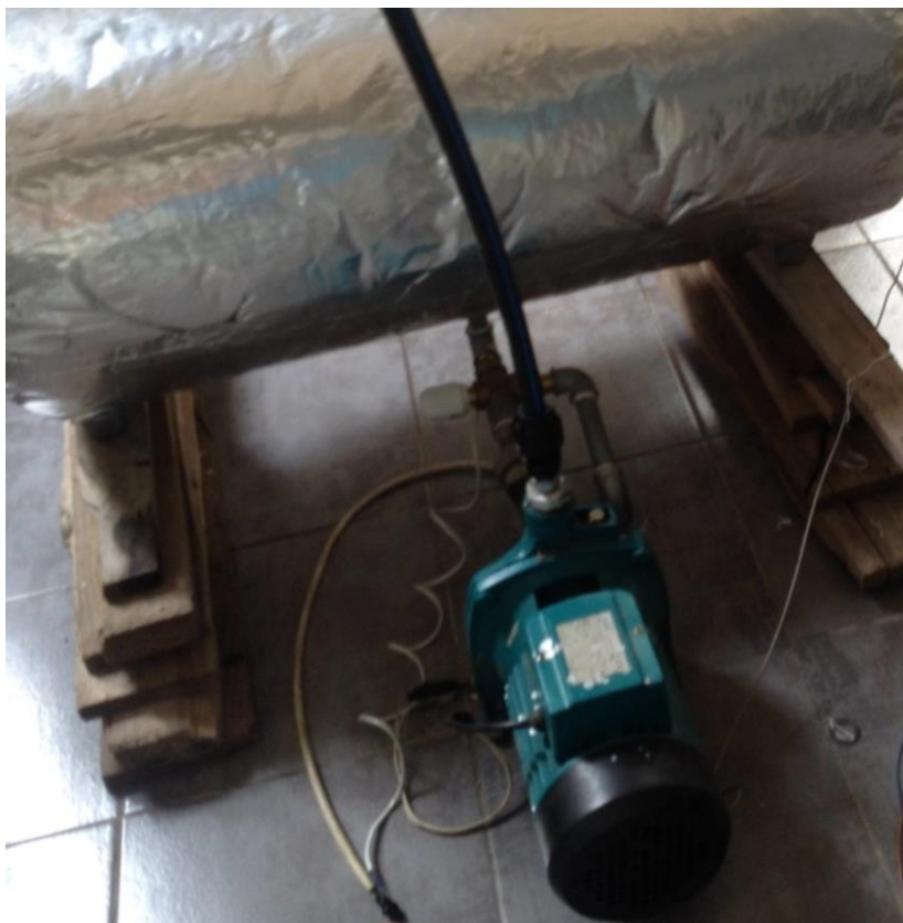
Figure 3.2: The test 2 concerning open/close valve turn on/off pump.
