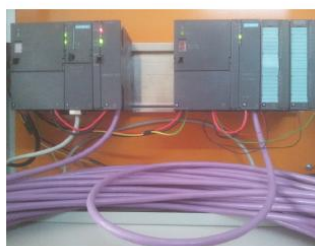
PLC System for MEGBI-VPP downstream processing system: Siemens S7-300 with PROFIBUS
