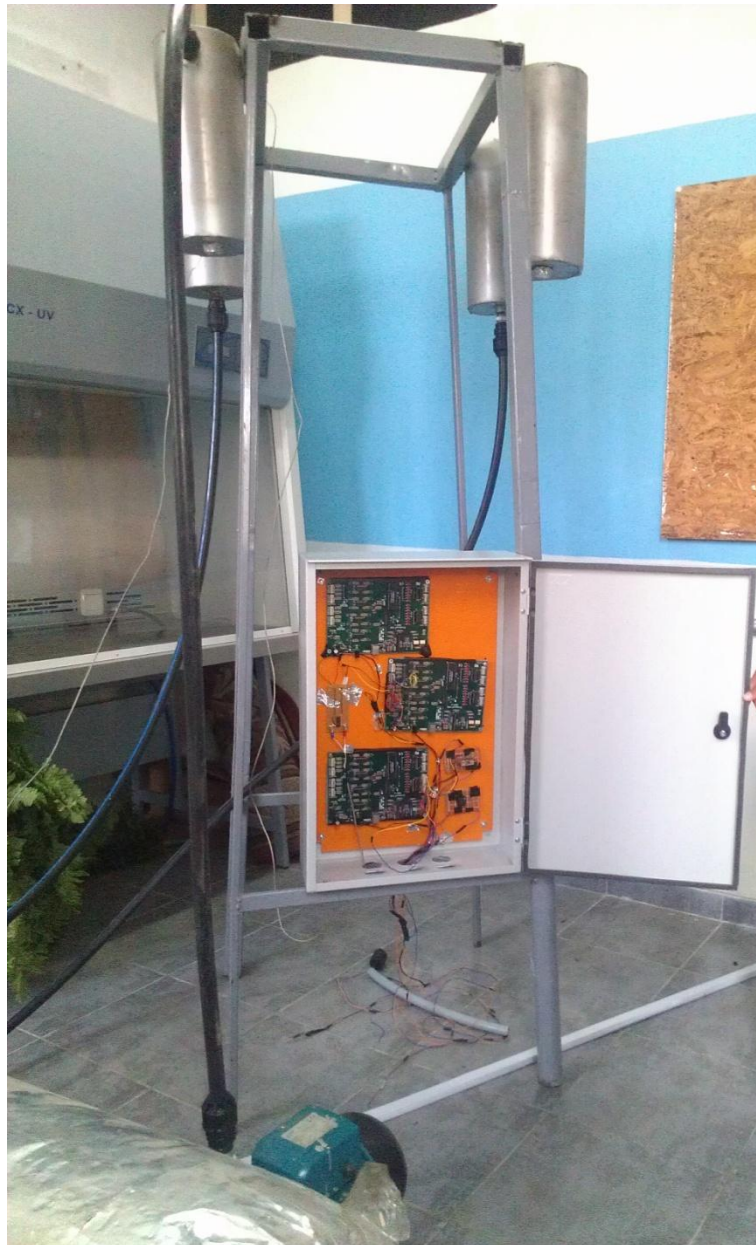
Figure 6.14b: Installed Electrical Control Cabinet
