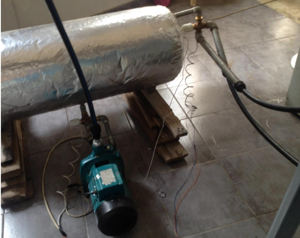
Figure 3.3: The Test 3 concerning open/close 2 valves and turn on/off pump.
