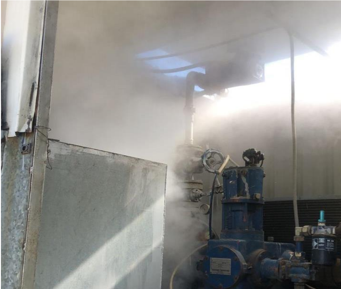
Stage 15 Steam leakage under the turbine (between the condenser and the turbine)
