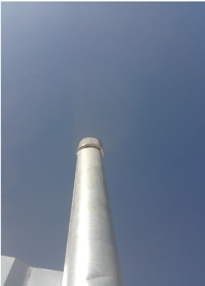
Figure 25: chimney during incineration
