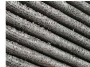
Fouling of Finned Tube Coils
