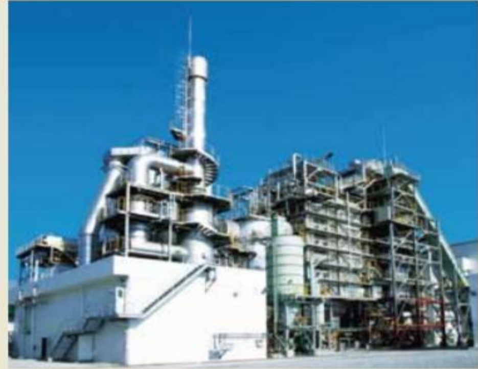
In Thailand, an industrial waste incinerator has been operating from 2006. Its treatment capacity is 100t/day. Source: JFE Engineering Corporation
