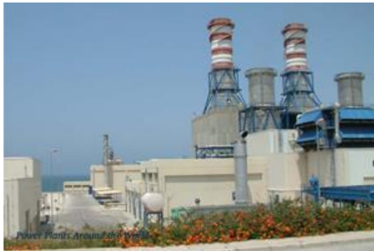
Deir Ammar power plant
