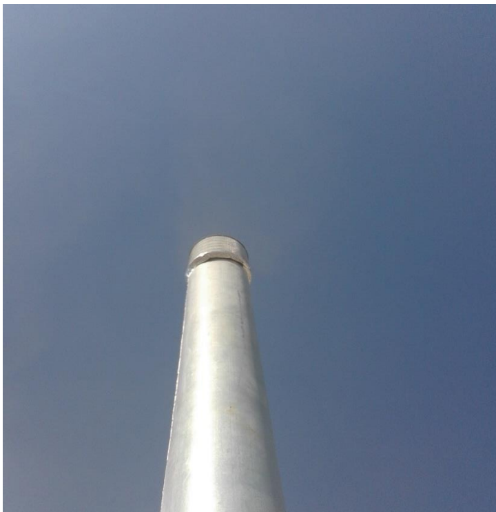
Figure 79:chimney during incineration
