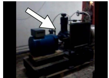
Successful test of turbine
