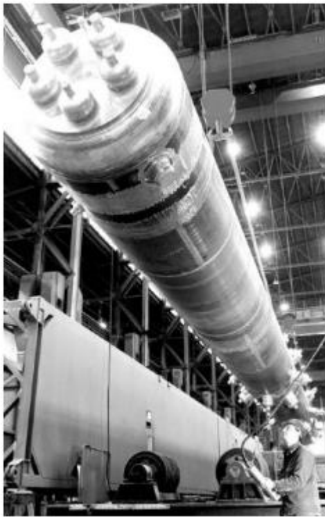
SWHE Installation into Cold Box
