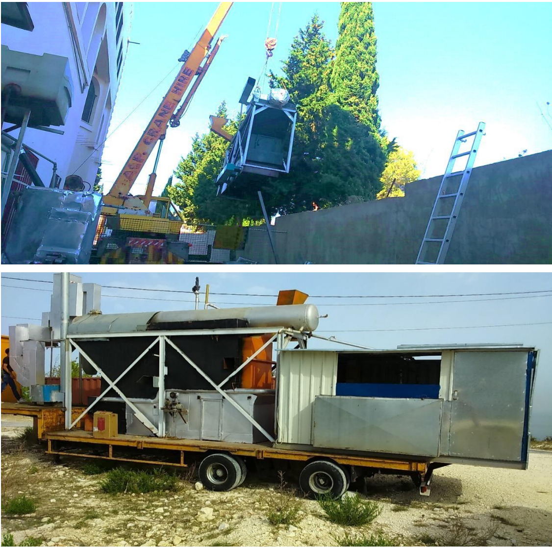
Figure 66: incinerator on mobile platform
