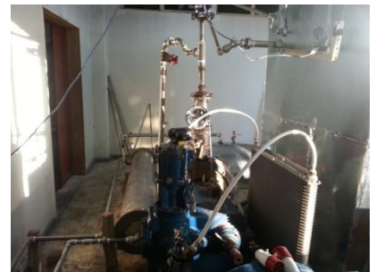
Integration of test rig
