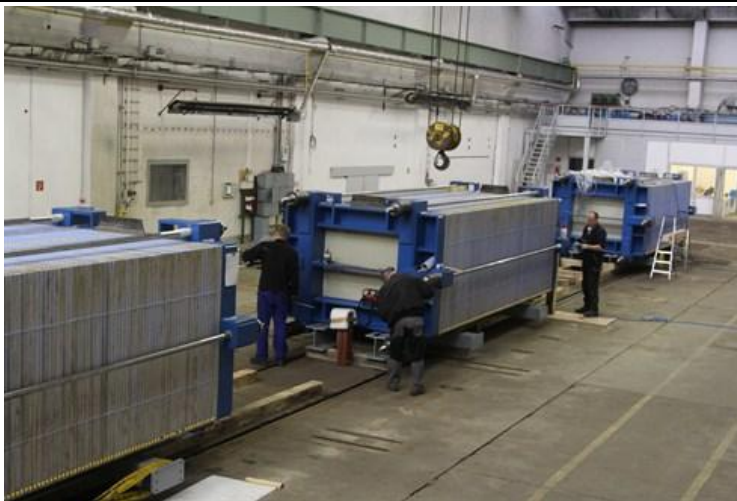
Figure 8: Three units of 2 MW Enertrag alkaline electrolysis unit - 1000 m 3 / h
