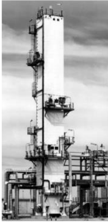
The SWHE Cold Box
