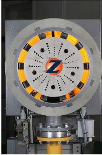
large natural gas burner.
