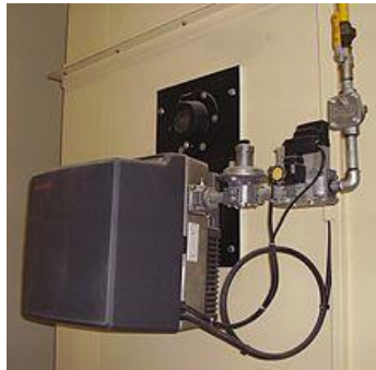
Burner with natural gas equipping an industrial cooking oven.
