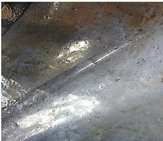
Figure 80:dust in silo with H 2 O condensed
