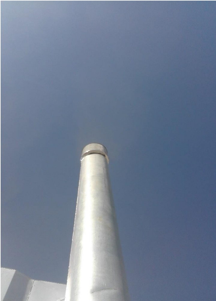
Figure 79:chimney during incineration
