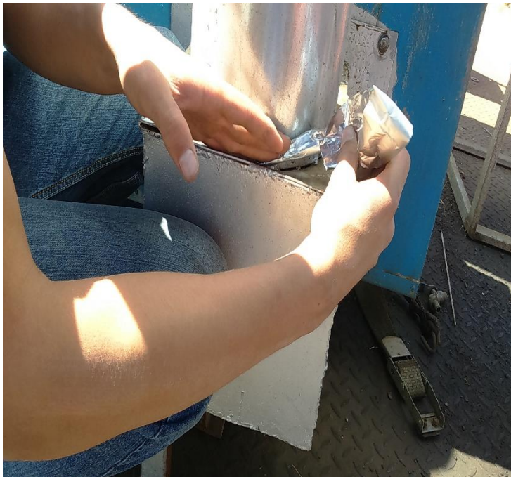
Figure 76: Closing the pores that leak fumes
