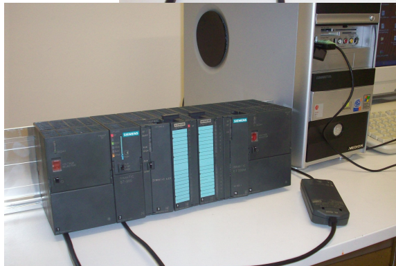
The Siemens S7 S300 for the TEMO-STPP test rig
