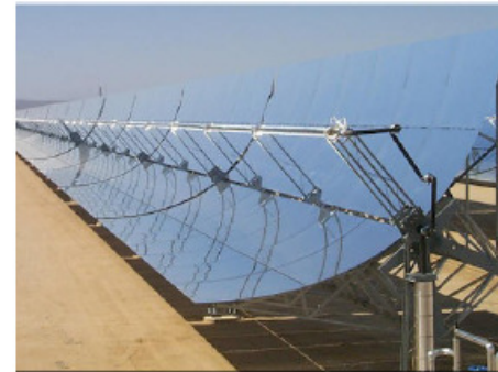
STPP test plant
