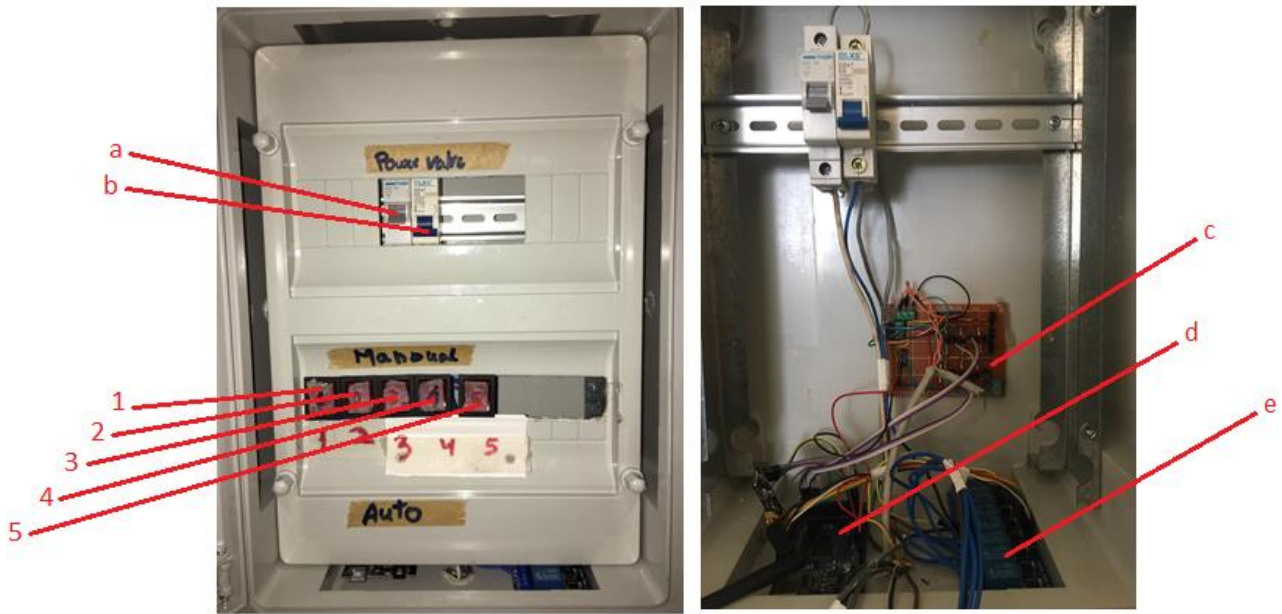
Fig.2. Power Control Box
