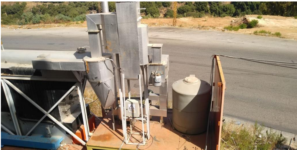
Figure 17 the power plant
