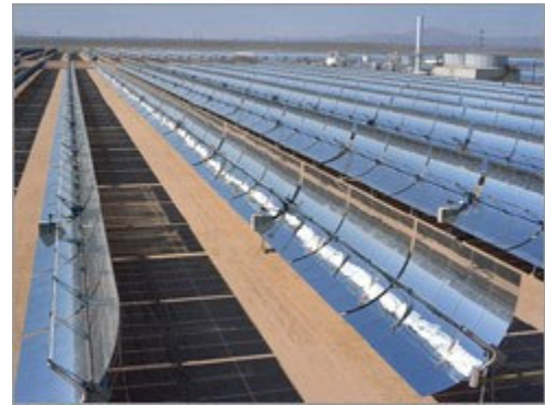
Solar collector array
