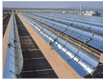
Solar collector array
