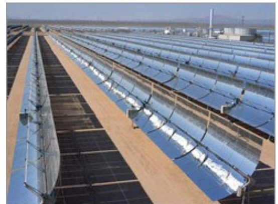
Solar collector array
