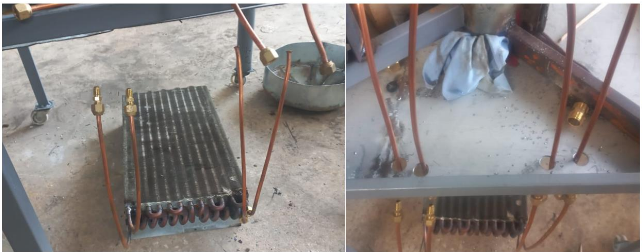
Picture 10 : Gasifier and Connecting Lines
