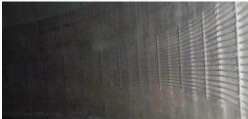
Digester heating system
