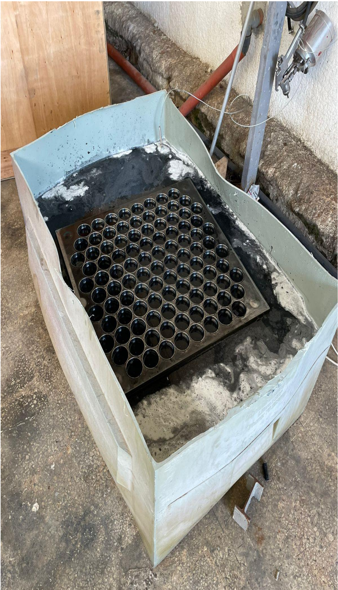
Here is how our cleaning of the Electro-Filter was done
