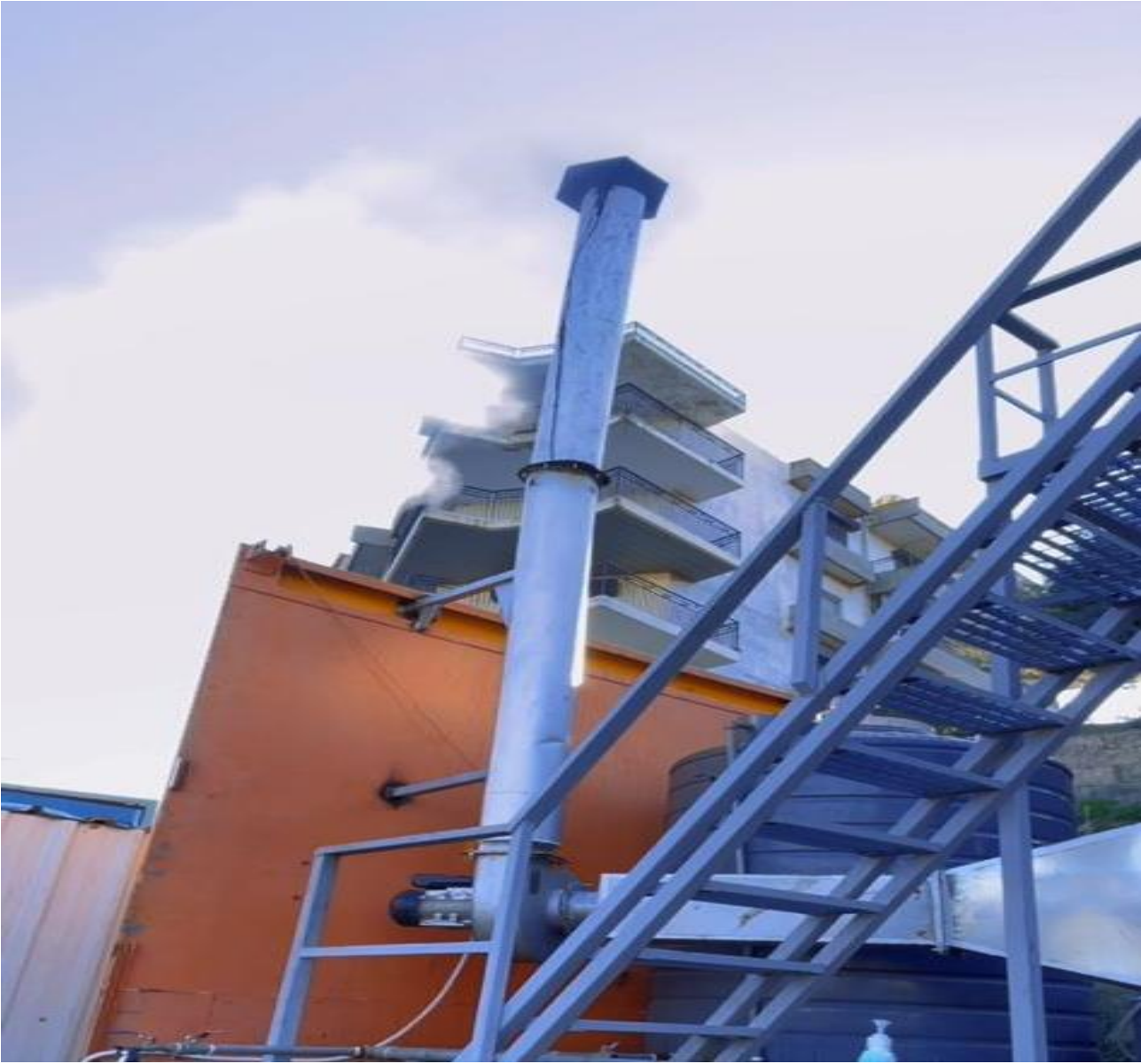
Flue gas getting out through the chimney pic
