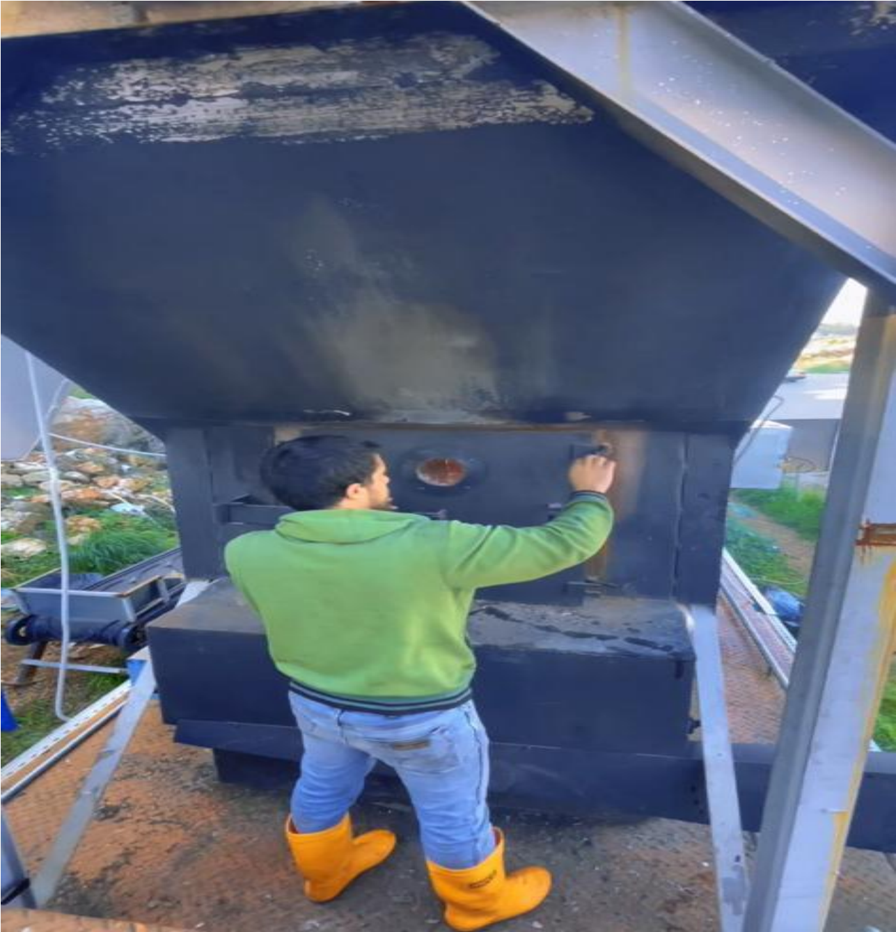
Incinerator chamber main gate pic
