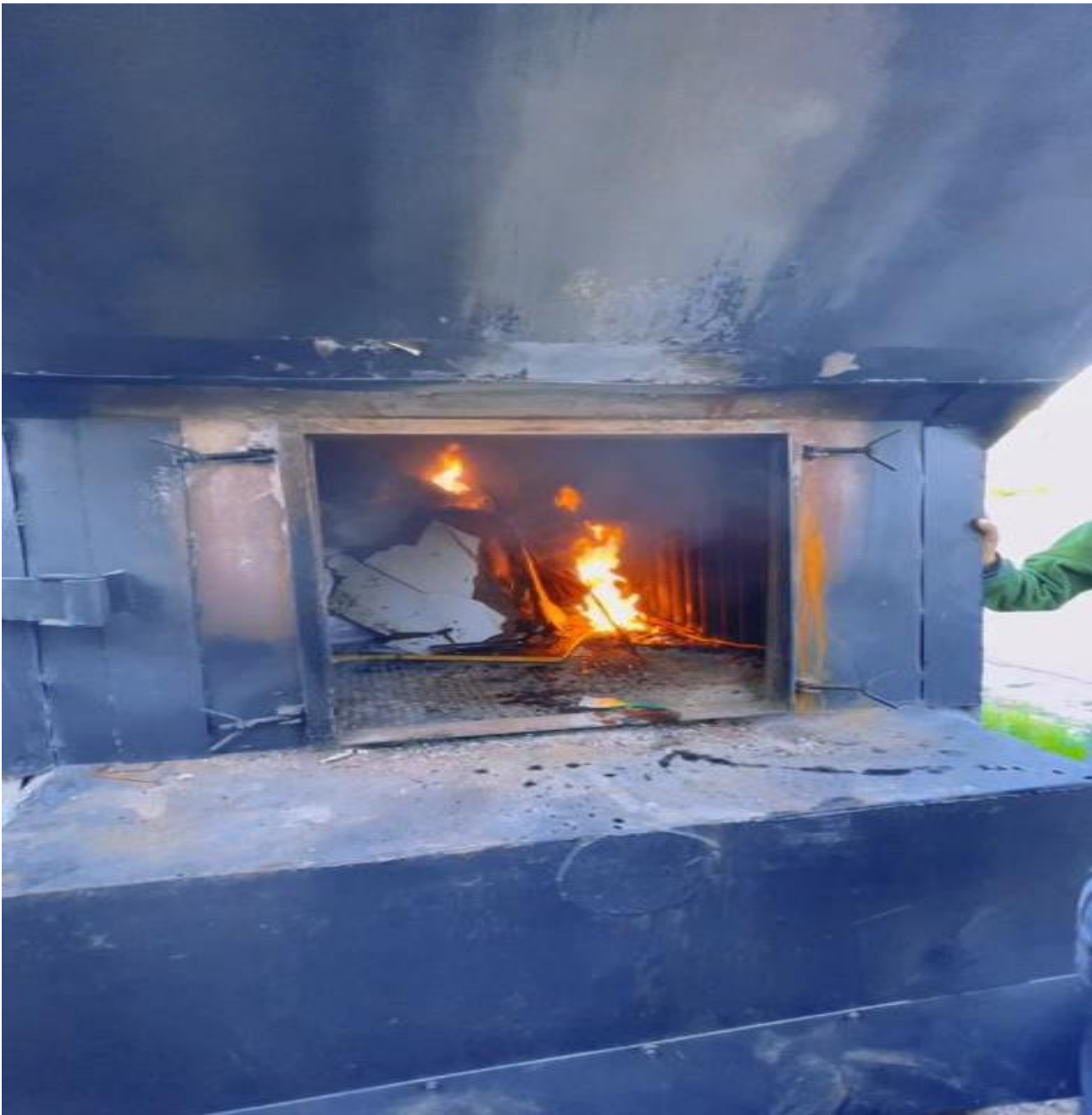
Incinerator chamber pic
