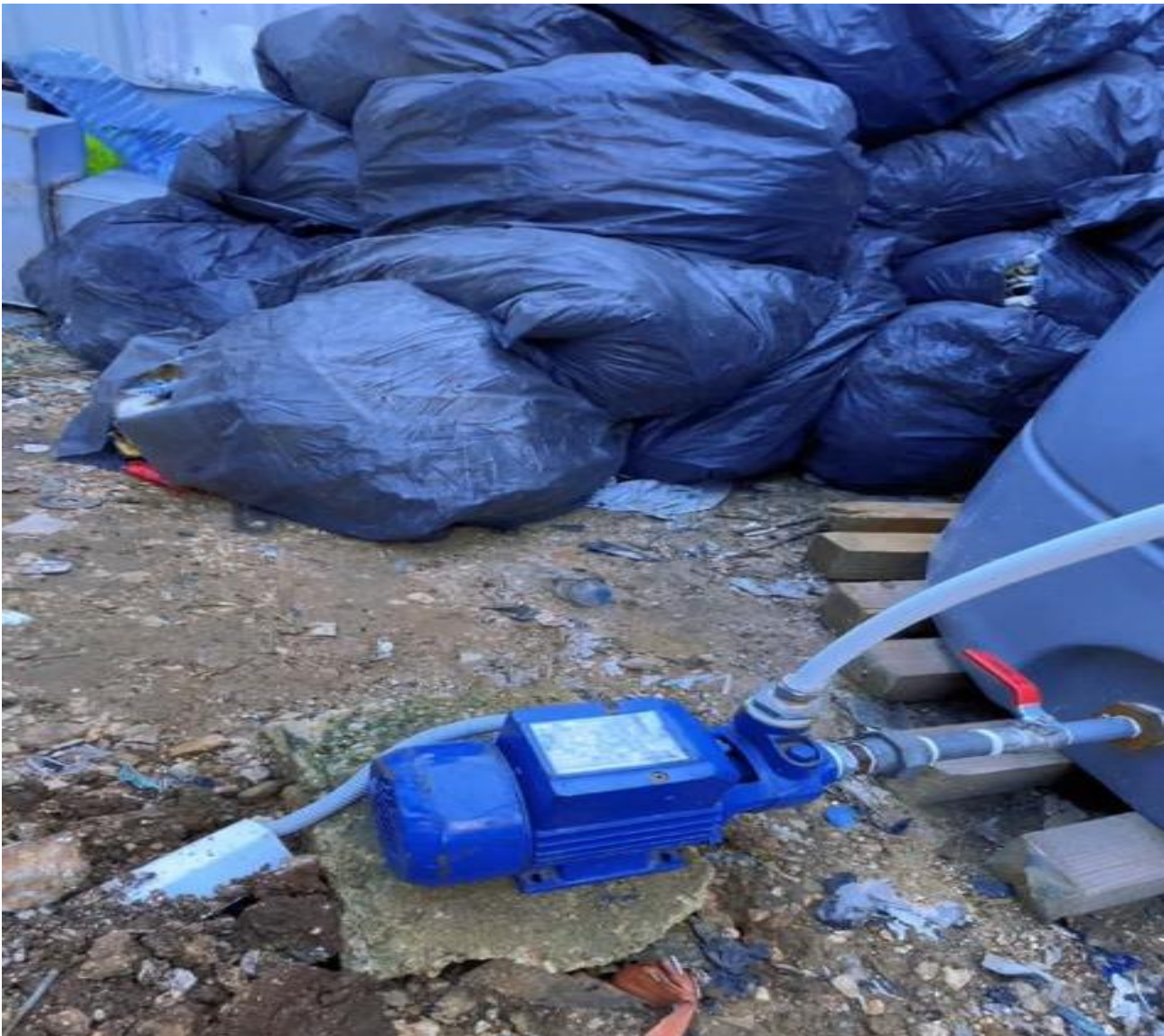
Water pump P1 pic
