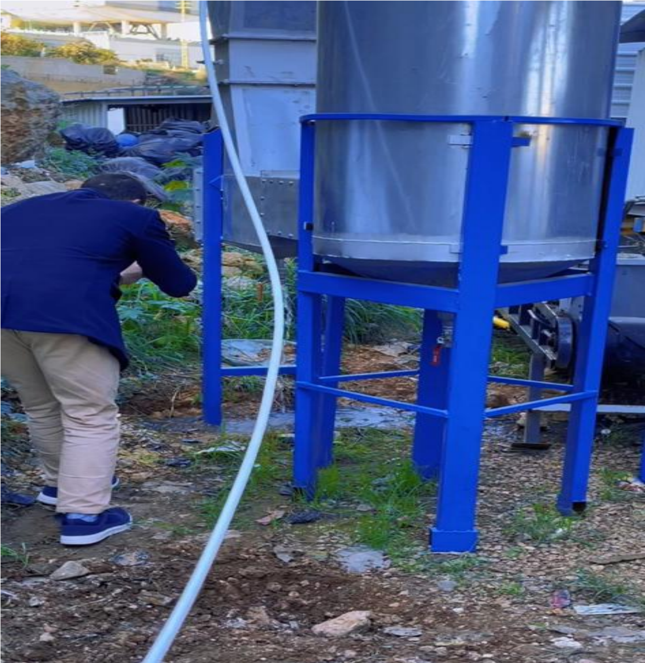
The drainage of the water by the scrubber cooler pic
