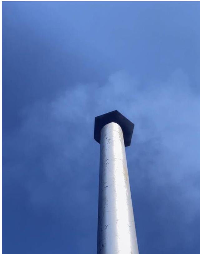
Before turning on the electro filter
