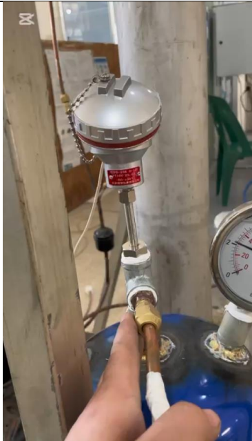
Exit of separator
