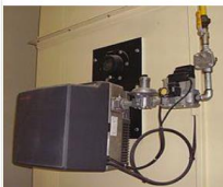
Natural gas burner equipping an industrial cooking oven
