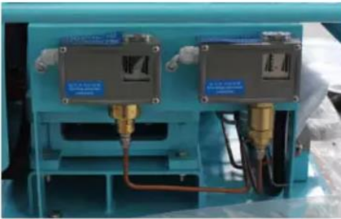
suction pressure switch discharge pressure switch
