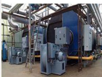
Combustion fan with frequency variator for gas / oil burners
