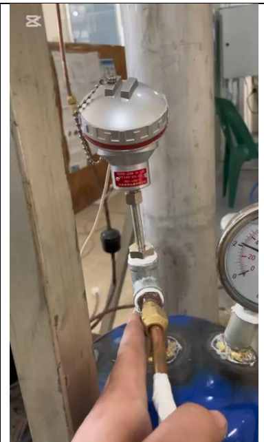
Exit of separator
