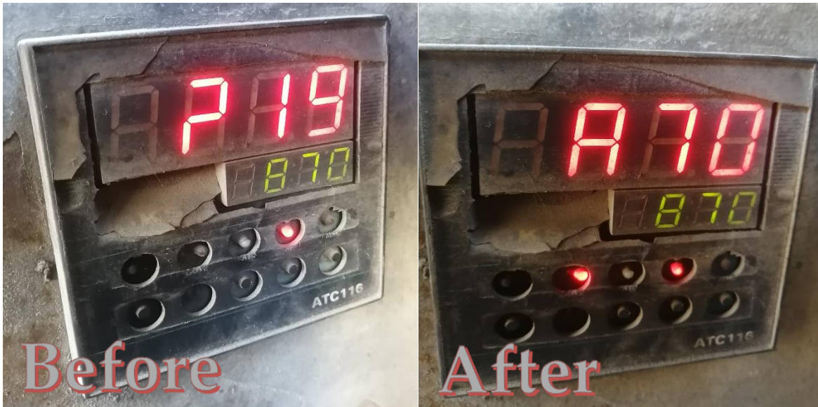
Figure 38: Numerical panel shows the temperature inside the furnace
