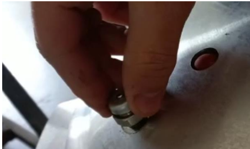
Figure 9-51. safety valve closed
