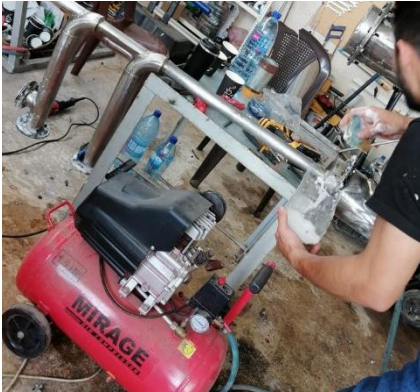
Figure III. 5: Carrying out a new check for the presence of air leaks
