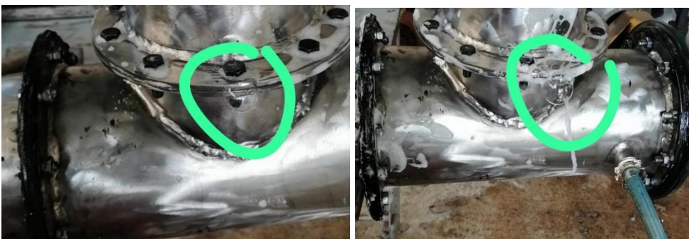
Figure III. 6: air leak locations
