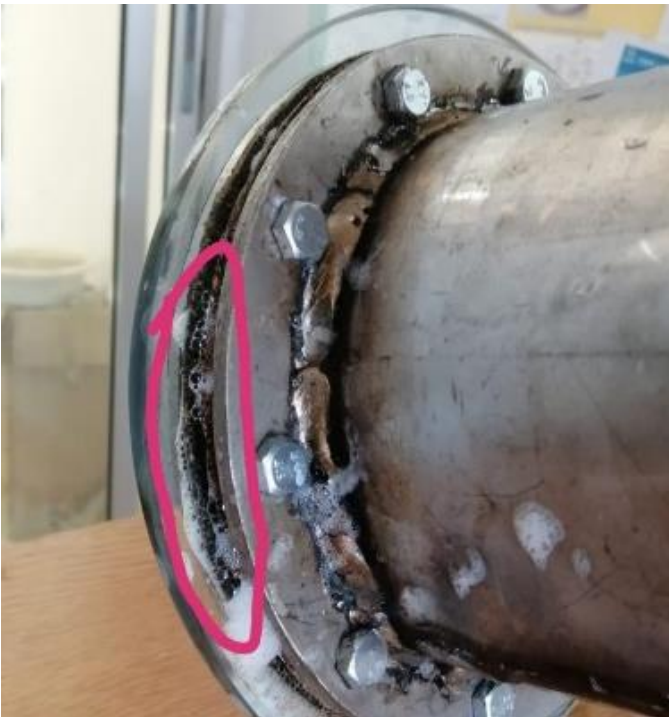
Figure III. 2: Air leak locations
