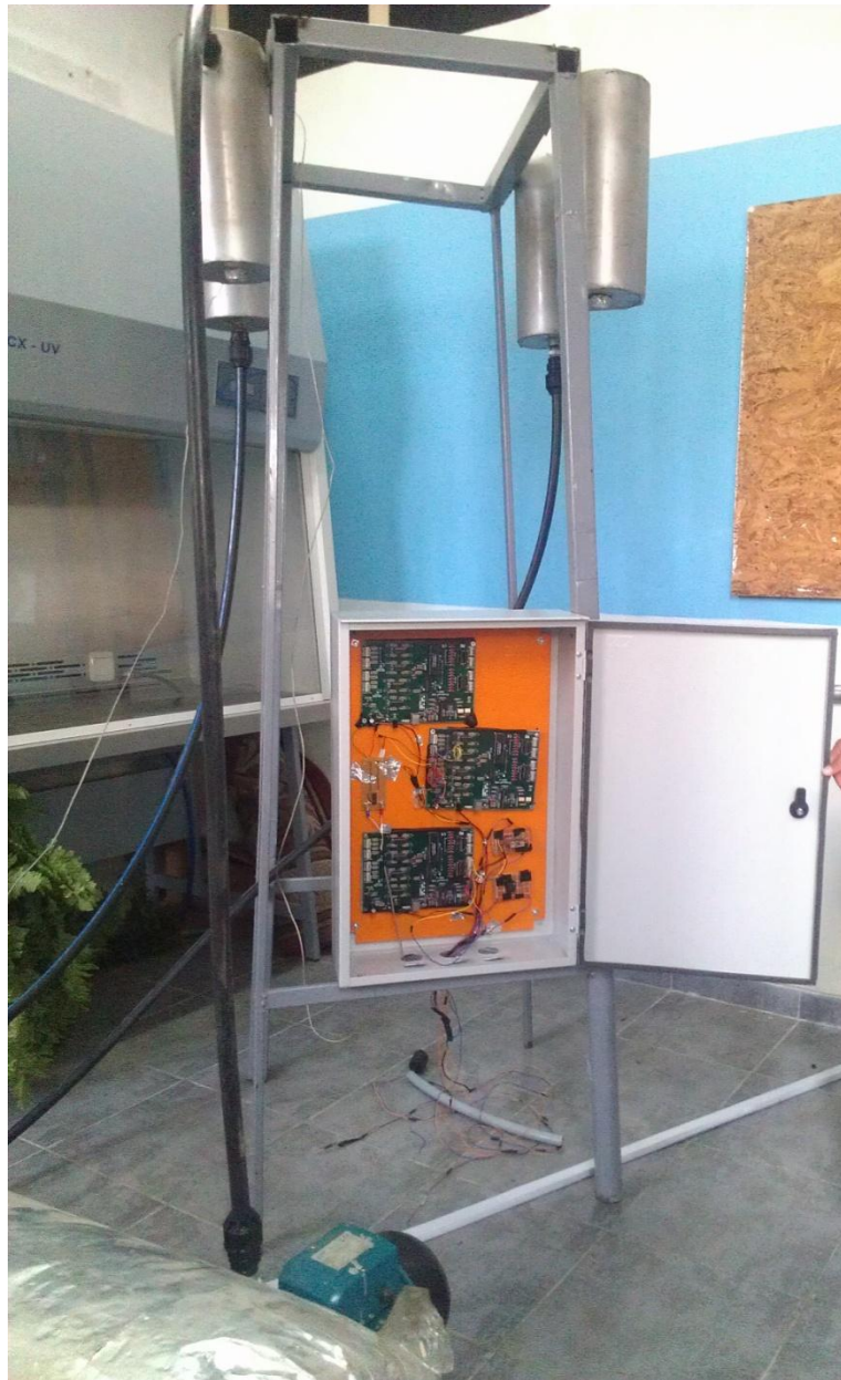
Figure 6.14b: Installed Electrical Control Cabinet
