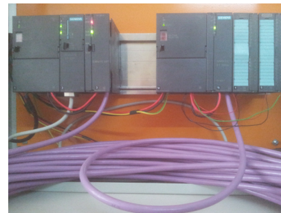
PLC System for MEGBI-VPP downstream processing system: Siemens S7-300 with PROFIBUS
