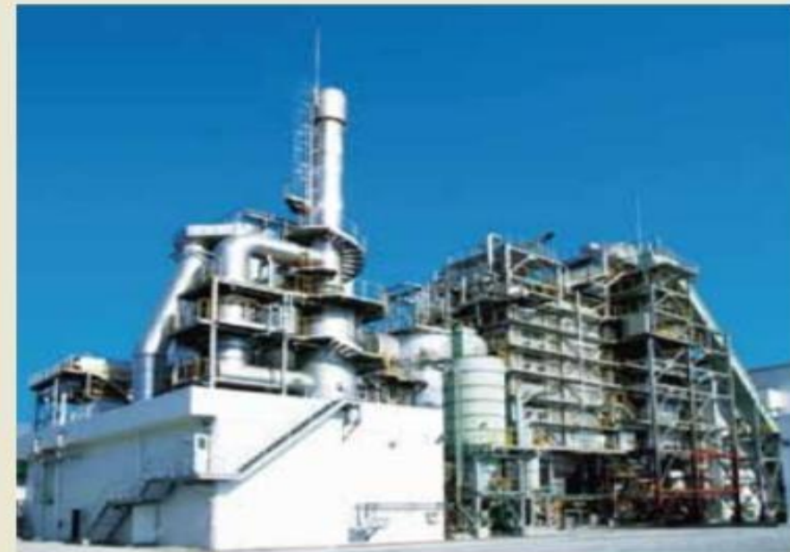
In Thailand, an industrial waste incinerator has been operating from 2006. Its treatment capacity is 100t/day. Source: JFE Engineering Corporation
