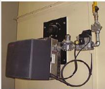
Natural gas burner equipping an industrial cooking oven
