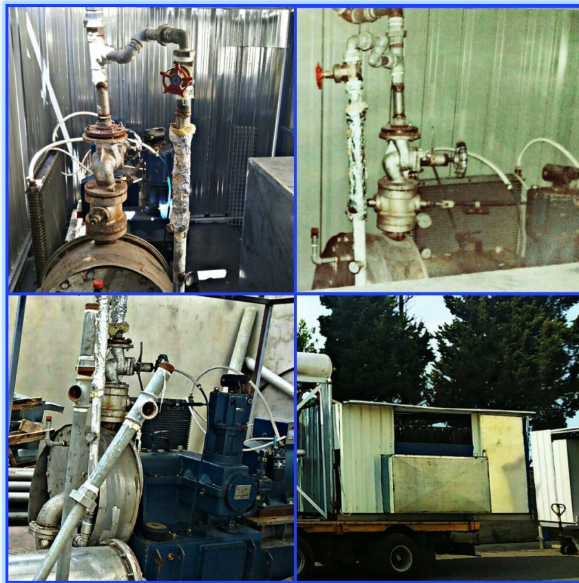
Figure 13: Steam turbine of 40 kW in North Lebanon Power Plant Company
