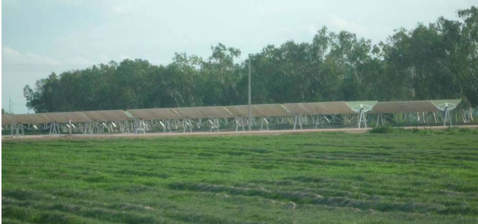
Fig. 2. Collectors at the KTSE-9100 Power Plant 4
