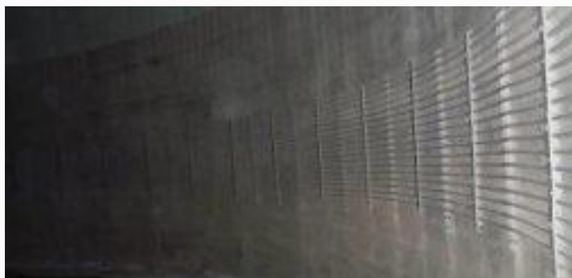
Digester heating system
