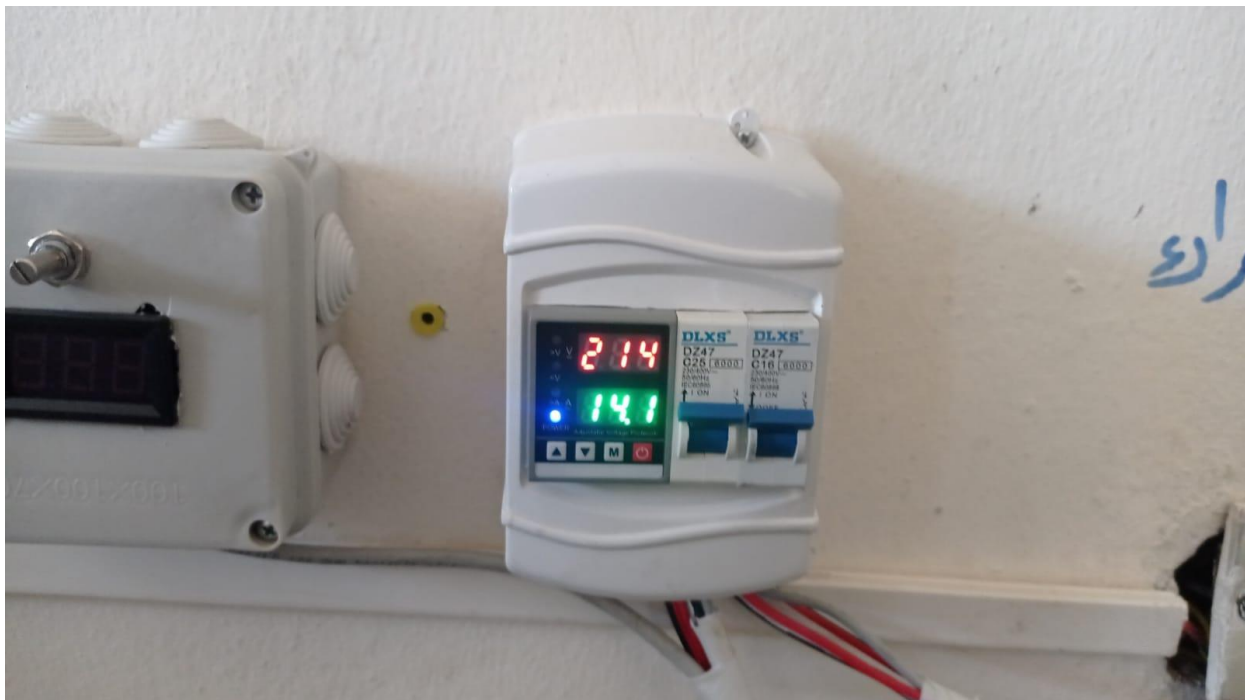
Fig. 3: Just after starting the machine (1A is going to the transformer)
