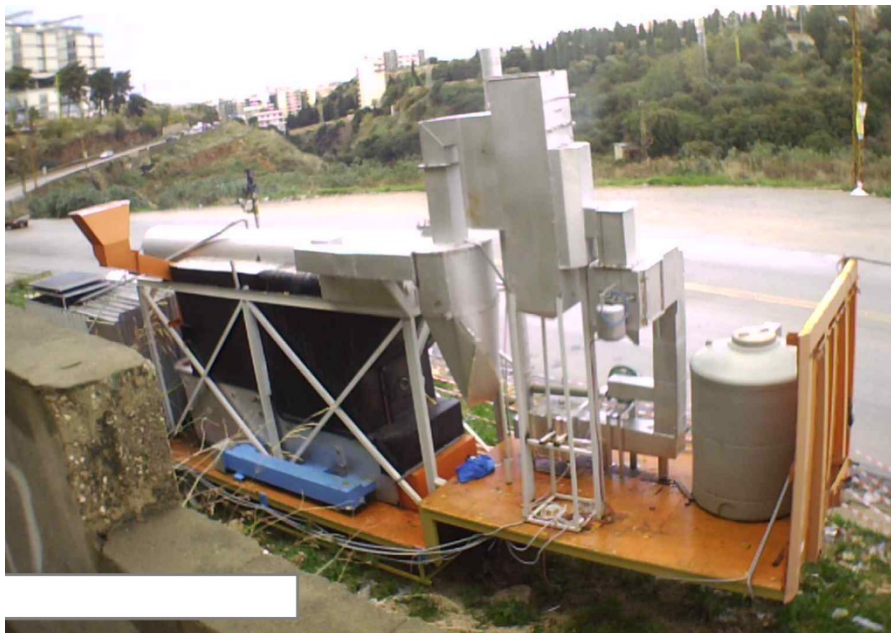
Figure 1.1: Real picture of a waste incineration power generation device
